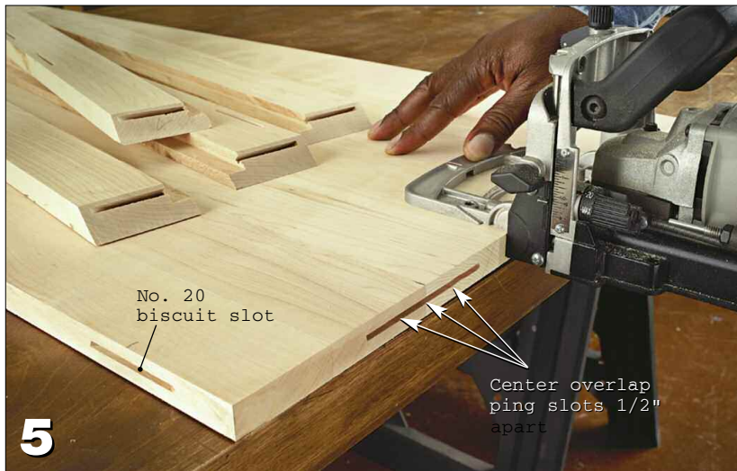
5 Cut three No. 20 biscuit slots in the side frames (see drawing for details), and then cut three overlapping biscuit slots to form elongated slots in the maple top side edges.
